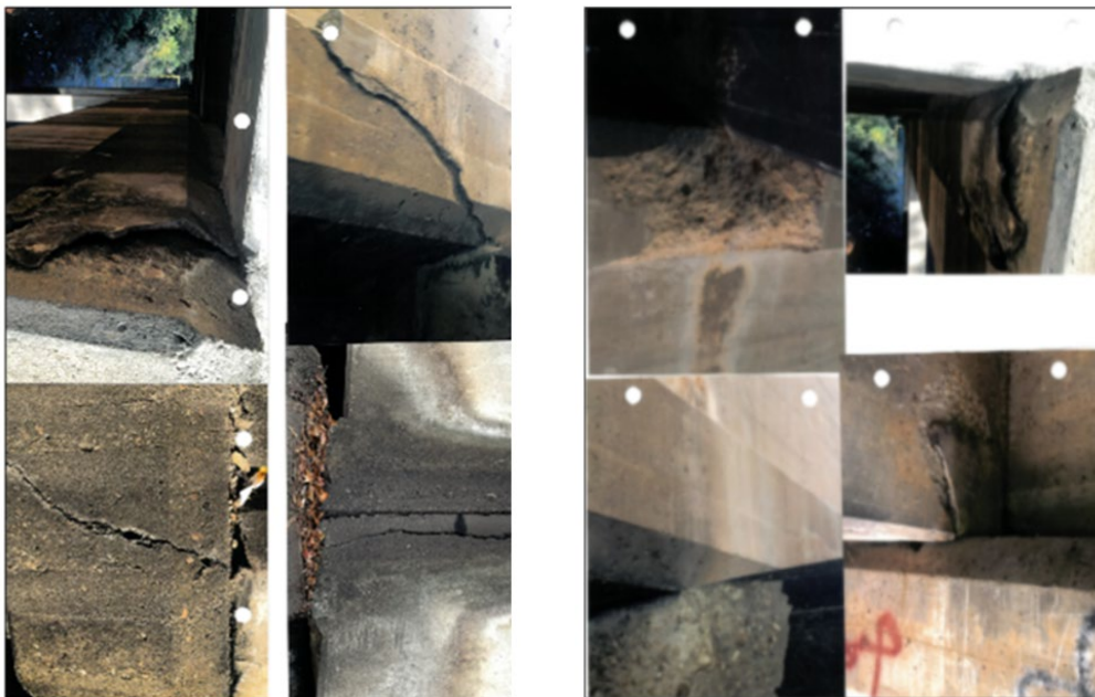
Figures 5 and 6. Deteriorated condition of the Stillman Boulevard Bridge
